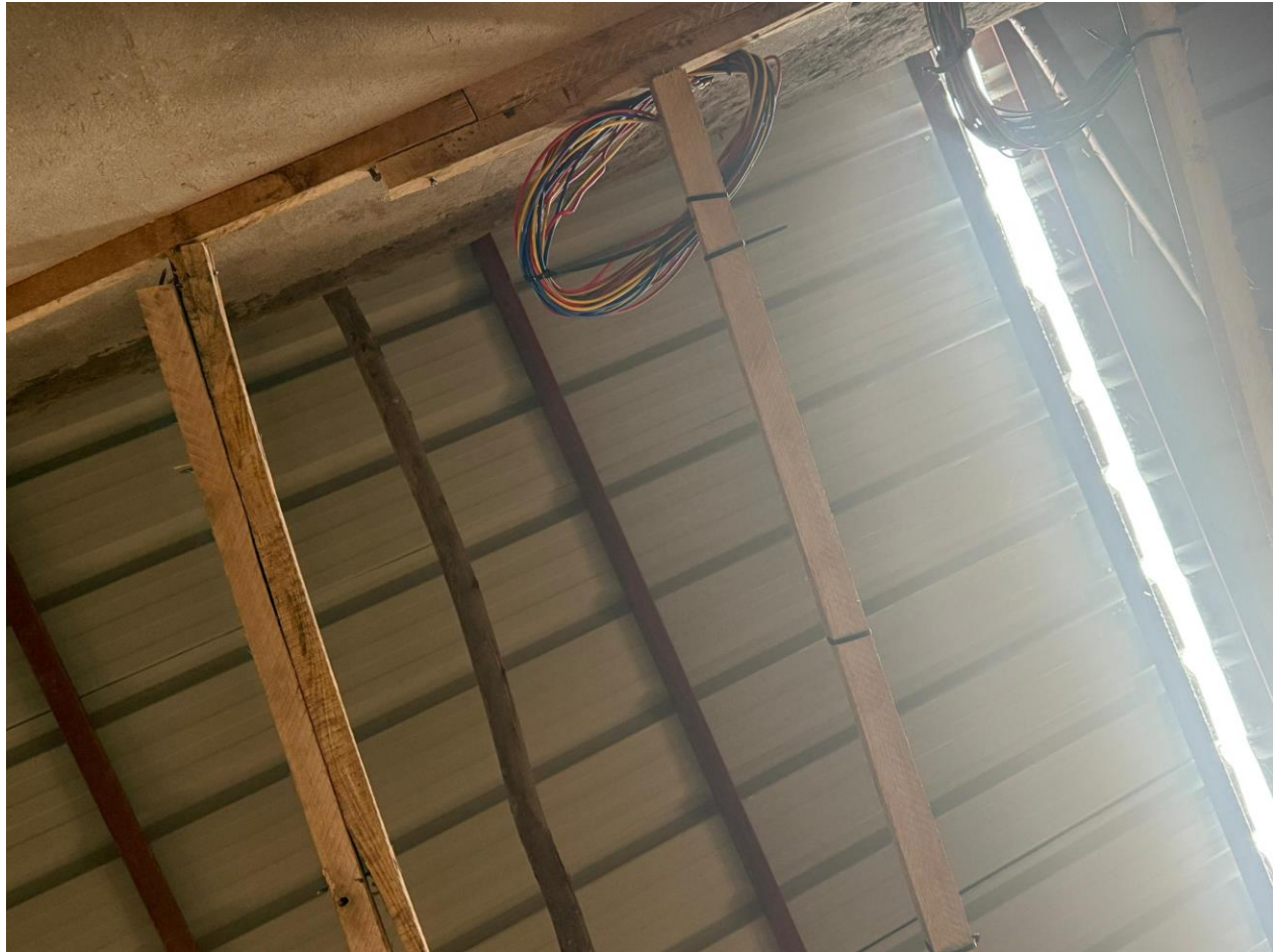
Figure 7: Electrical wiring cable
