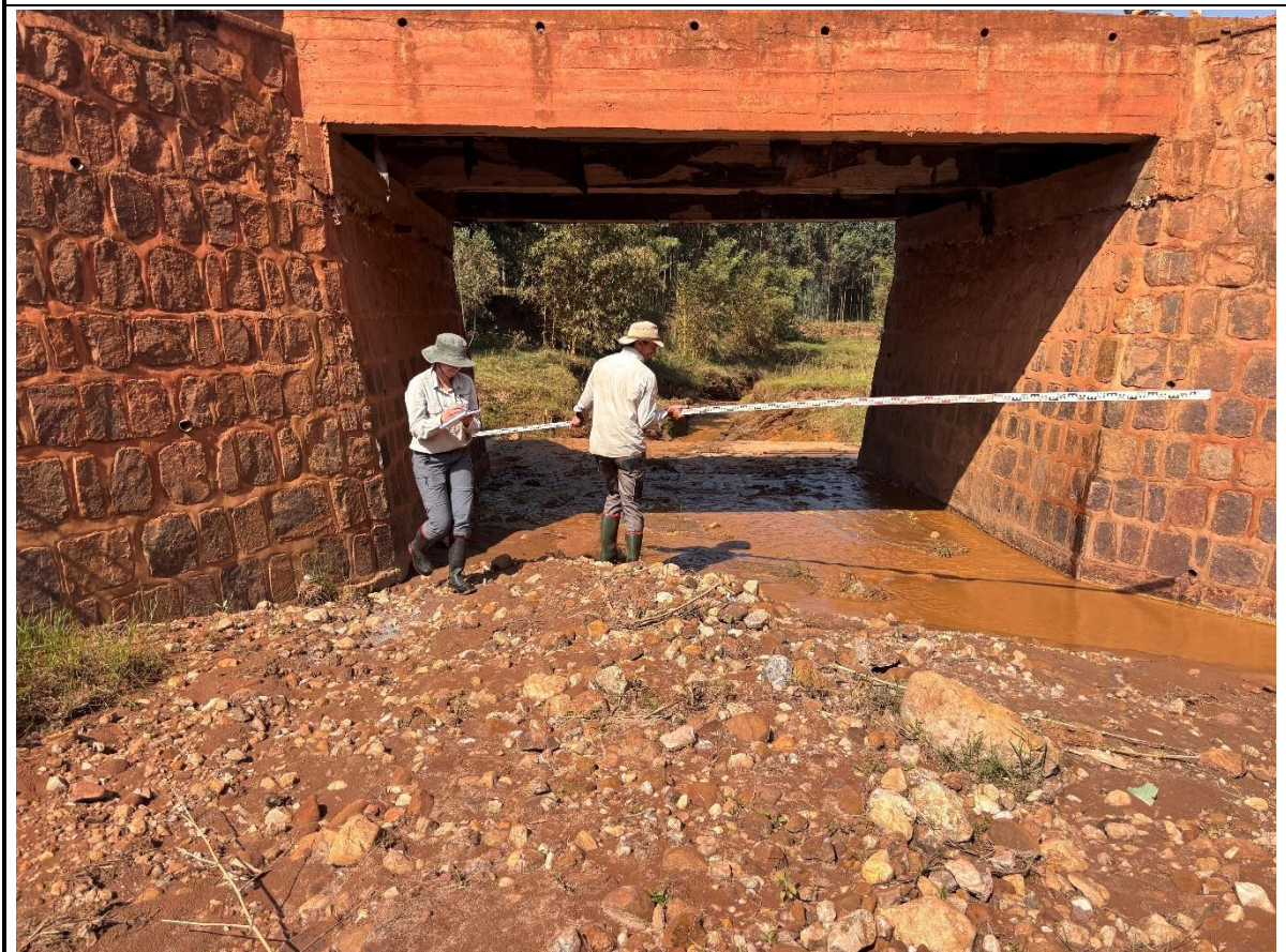
Photograph showing team members measuring the dimensions of hydraulic infrastructure. The length, width, height and invert level of the bridge culvert was surveyed.
