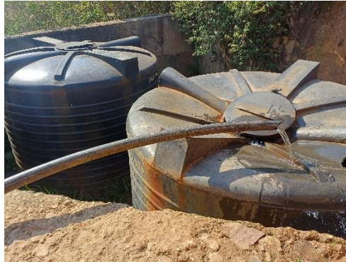
Storage tanks at the mine pumphouse
